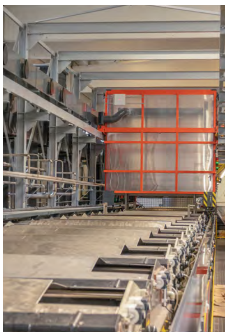
(right) The Costa Trattamenti completely automated metal treatment plant, Brescia, Italy
